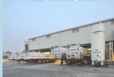
Existing helium center
