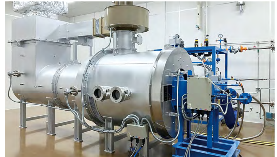
Mixed hydrogen combustion and oxygen-enriched combustion equipment at the Iwatani R&D Center
