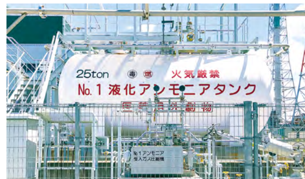
An ammonia supply facility
