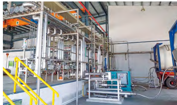
New refrigerant filling equipment (Thailand)
