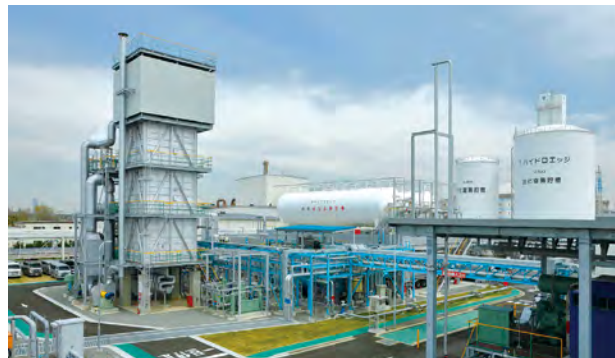
Hydro Edge liquid hydrogen production plant
