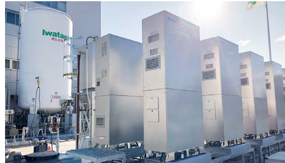
Pure hydrogen fuel cells (20 5 kW cells) adopted at the Iwatani R&D Center
