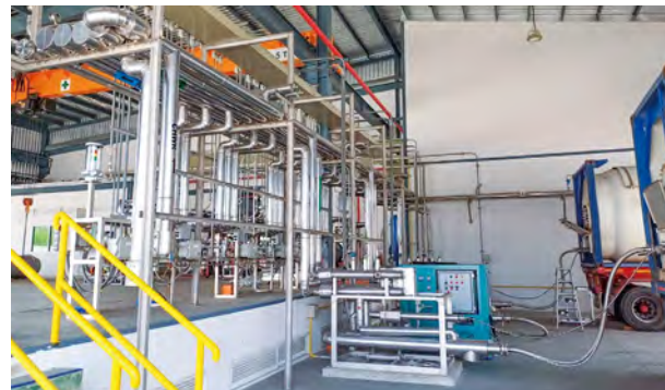
New refrigerant filling equipment (Thailand)
