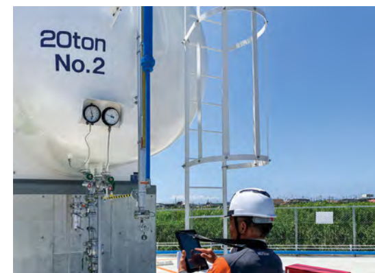
Plant equipment maintenance using a tablet
