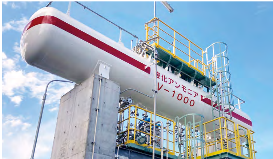
Liquefied ammonia tank for mixed combustion with ammonia
