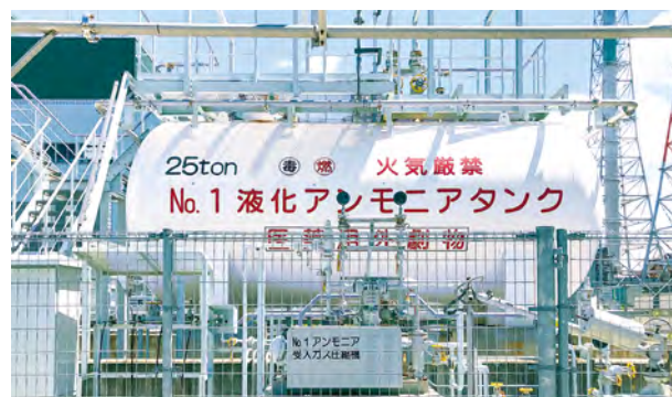
An ammonia supply facility
