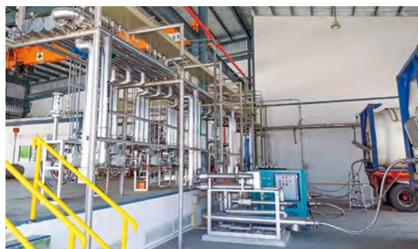
New refrigerant filling equipment (Thailand)
