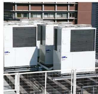
GHP (Gas Heat Pump) air conditioning system
