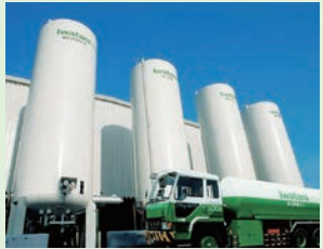
High-pressure gas supply facilities
