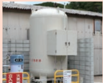
LPG supply equipment
