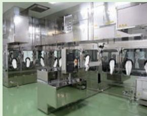
Pharmaceutical manufacturing equipment
