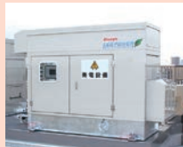
LPG-powered emergency generator
