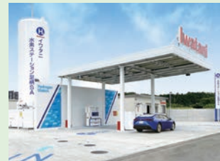
Hydrogen-refueling station equipment
