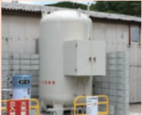
LPG supply equipment
