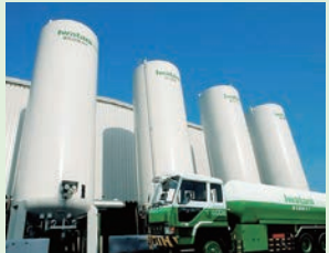
High-pressure gas supply facilities
