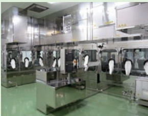
Pharmaceutical manufacturing equipment
