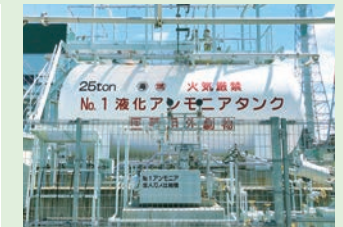
Ammonia supply equipment
