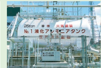
Ammonia supply equipment
