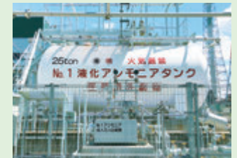
Ammonia supply equipment
