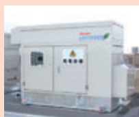
LPG-powered emergency generator
