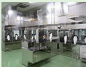
Pharmaceutical manufacturing equipment
