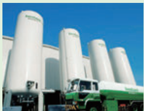
High-pressure gas supply facilities
