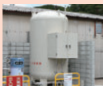
LPG supply equipment
