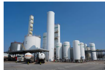
Air separation plant (Jiaxing, China)
