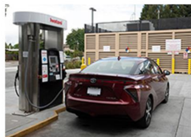
Iwatani Mountain View H2 Fueling
