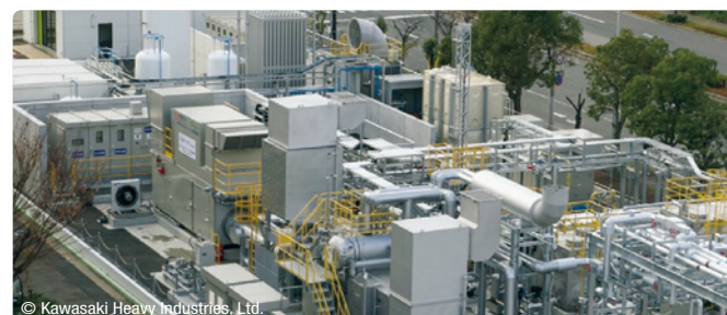
Photo of the Kobe Smart Community Hydrogen Power Generation Project (Port Island), a NEDO subsidized project (undertaken by Obayashi Corporation and Kawasaki Heavy Industries, Ltd.)
