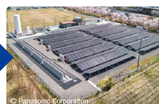
H 2 KIBOU FIELD (Kusatsu facility, Panasonic Corporation)
