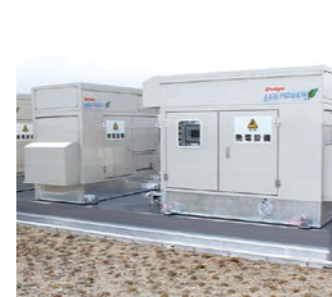
LPG-powered emergency generators
