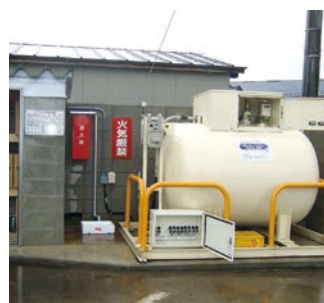
Disaster-ready LPG bulk storage tank
