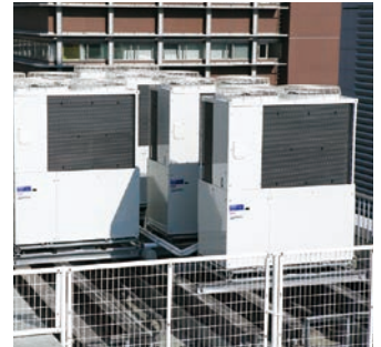
GHP (Gas Heat Pump) air conditioning system
