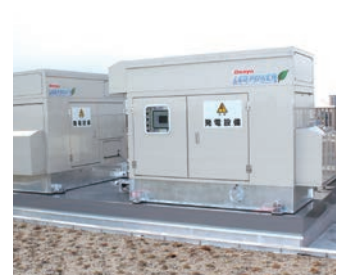
LPG power emergency generator
