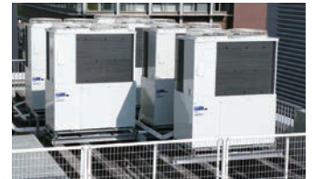
GHP (Gas Heat Pump) air conditioning system
