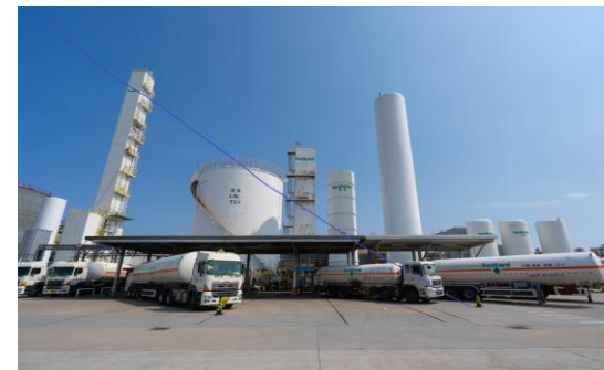
Air-separation gas unit of Jiaxing Iwatani Industrial Gases Co., Ltd.
