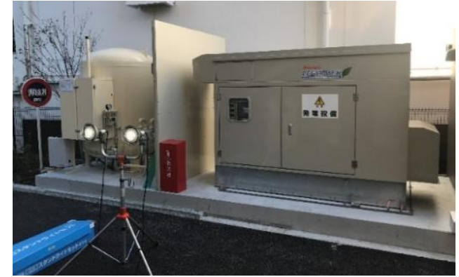
Emergency LPG generator and bulk storage
