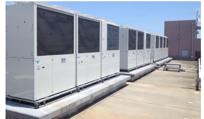
GHP (gas heat pumps)
